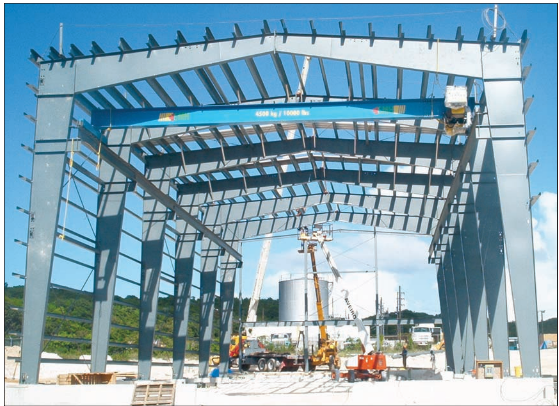
Figure B1: Top Running Crane
